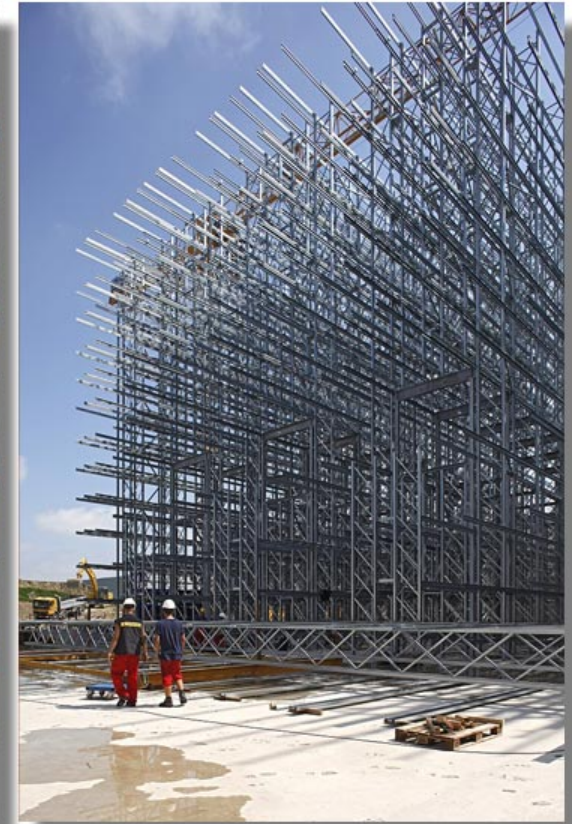
Deep freeze store of Pistor, Switzerland. (70m long and 35m high)
